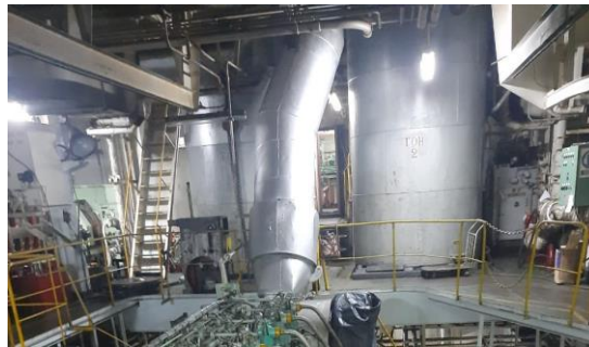
Gambar 4. Main Air Compressor
