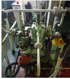
Gambar 3. Main Air Compressor
