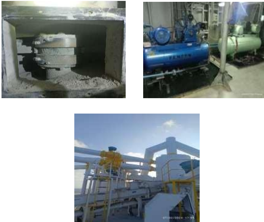
Picture 1. compressor and unloading screw Which connected with system pneumatic.
